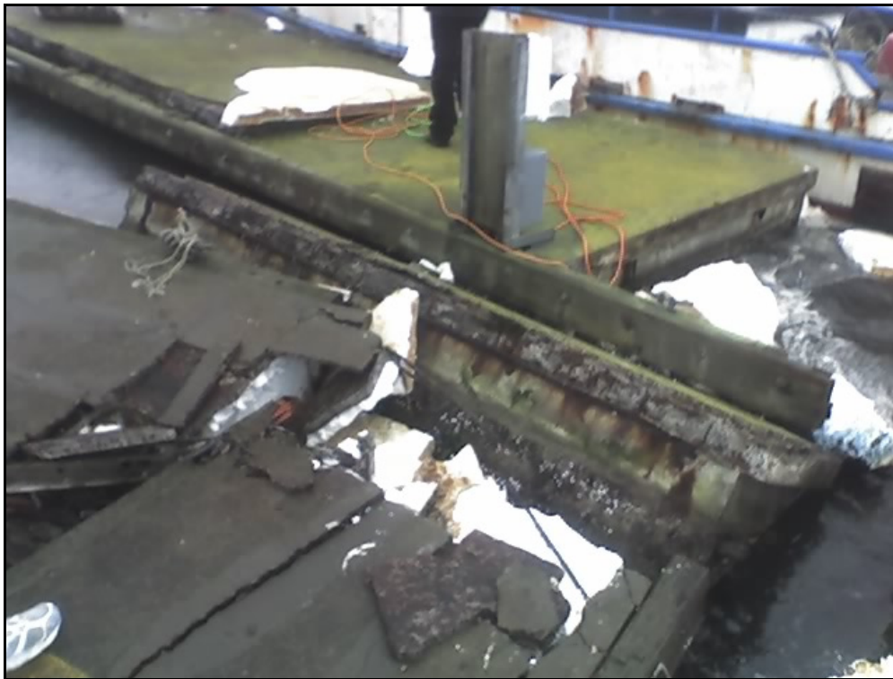
Photos of Damage to Crescent City Harbor.
