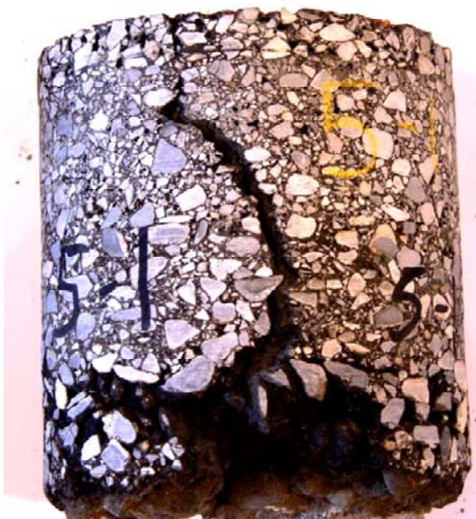
Figure 11-3 The UTACS cracks remained the same width all through-out the core, except at the membrane which remained sealed although the crack had reflected to the surface (Sebaaly, 2007).
