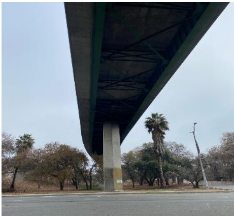
Photo 19. Habitat surrounding steel girder bridge with multiple expansion joints, and crevices along abutments, consists of landscaped lawns, mowed areas below bridge, residential/industrial buildings, and trees with clusters of dense leaf foliage and crevices for potential roost habitat (Location #37). Taken facing east.
