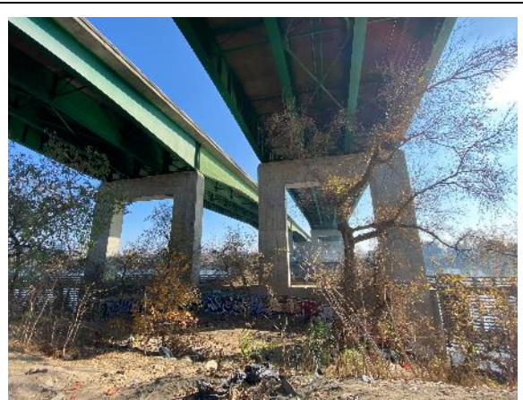
Photo 22. Steel girder bridge with multiple expansion joints, abutments with crevices spans the Sacramento River and leads to developed and disturbed area in Sacramento. Habitat surrounding the bridge consists of landscaped lawns, mowed areas below the bridge, residential and industrial buildings, homeless encampments, and potential tree roost habitat along the Sacramento River and urban street trees with dense clusters of leaves and crevices (Location #41). Taken facing southeast.
