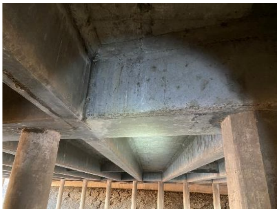
Photo 15. Signs of bat night roosting were observed throughout the bridge, including guano and staining spots along the bridge deck (Location #28). Taken facing east.
