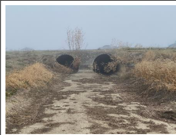
Photo 5. Multiple, large diameter corrugated steel culverts running below I-80 and adjacent frontage roads. Culverts below I-80 had signs of bat use, likely night roosting. (Location #5). Taken facing east.
