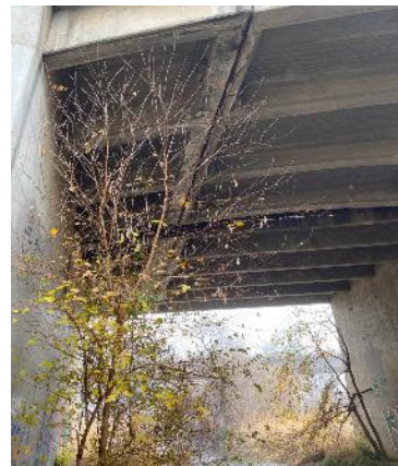
Photo 8. Bridge with multiple expansion joints along I-80 spanning the South Fork of the Putah Creek were occupied by Mexican free-tailed bats. Willow and cottonwood trees along creek provide suitable foliage roost for western red bat (Location #7). Taken facing north.
