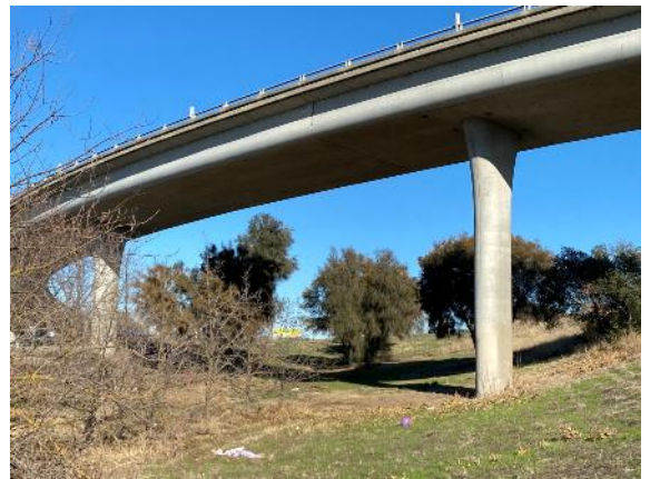
Photo 24. Habitat along multiple concrete box bridges with expansion joints consists of mowed annual grasses, industrial buildings, and potential tree roost habitat with dense clusters of leaves and some crevices, though most trees were small and unlikely to be occupied by bats, including some palm trees in adjacent to the bridges (Location #42). Taken facing east.
