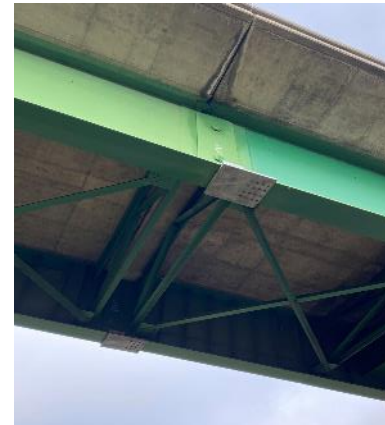
Photo 20. Bat guano was observed in crevices along the length of multiple expansion joints. Based on the amount of guano observed, the expansion joint could be occupied by a maternity colony during maternity season (Location #37). Taken facing northeast.
