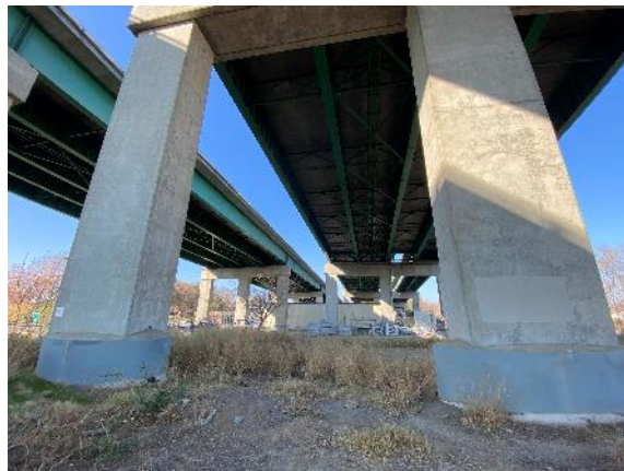
Photo 23. Potentially suitable bat roost habitat consists of steel girder bridge with multiple expansion joints and some crevices observed along the bridge abutments. Bat guano was observed in crevices of multiple expansion joints. Based on the amount of guano observed, the expansion joint could be occupied by a maternity colony during maternity season (Location #41). Taken facing northwest.
