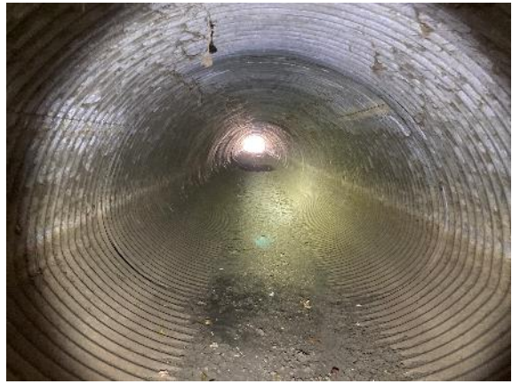
Photo 6. Multiple, large diameter corrugated steel culverts running below I-80 and adjacent frontage roads. Culverts below I-80 had signs of bat use, likely night roosting. Habitat surrounding bridge consists of perennial grasslands, orchards, and small stand of trees with clusters of dense leaf foliage and crevices for roosting bats (Location #5). Taken facing southeast.
