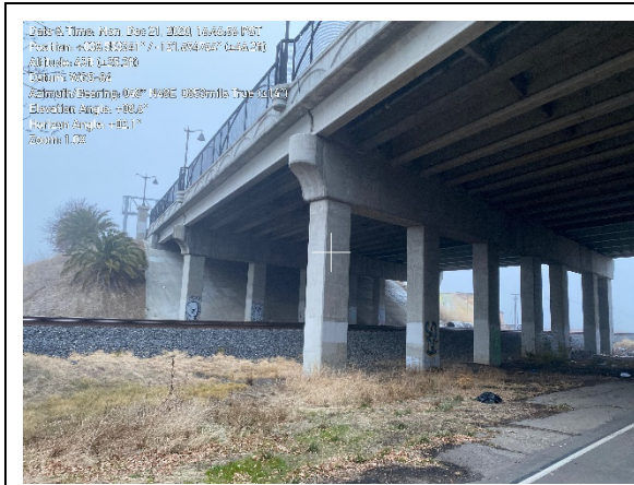
Photo 13. Habitat surrounding concrete girder/steel box bridge with expansion joints, utility boxes, bridge abutments (all potentially suitable bat roost habitat) consist of mowed annual grasses, industrial buildings, and potential tree roost habitat with dense clusters of leaves and crevices. (Location #25). Taken facing northeast.
