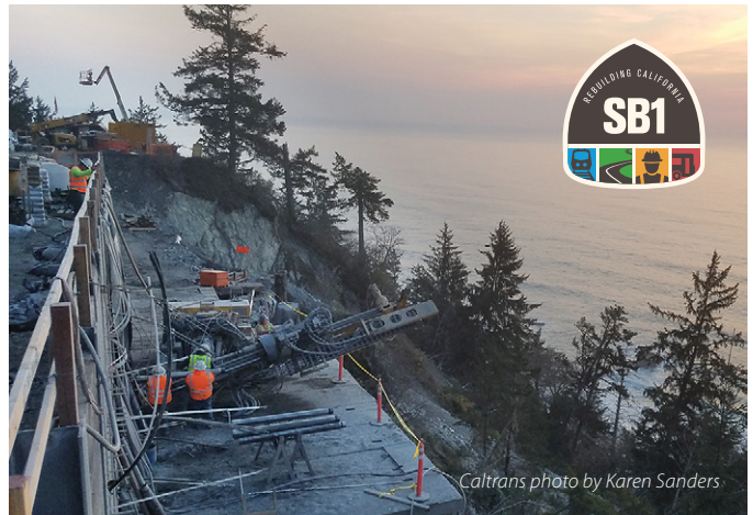
On US 101 in Del Norte County, crews perform repairs on the highway at what's known as Last Chance Grade south of Crescent City.
