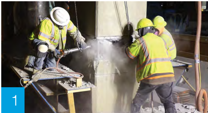
Once supports are in place, the concrete of the bridge columns is chiseled away to expose the steel rebar.
