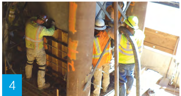
Concrete is poured into wood forms to create a new, taller bridge column.
