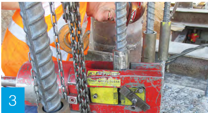
Bridge column reinforcement bars (rebar) are now separated by 16 to 21.5 inches. Steel couplers are used to reconnect the rebar inside each bridge column.
