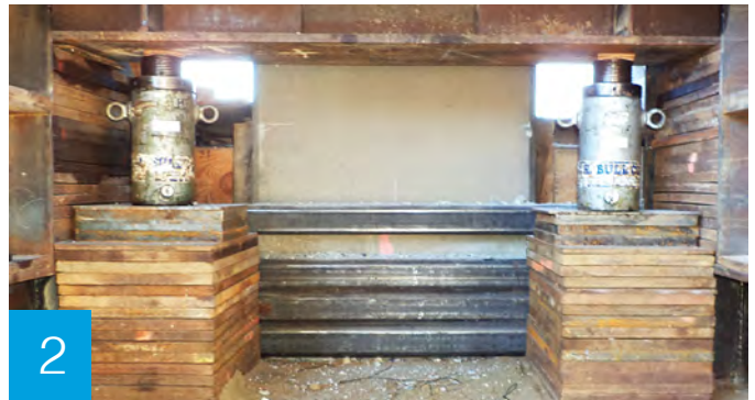
Hydraulic jacks, capable of lifting four to six inches, raise the steel frame that supports the bridge deck. Wood/steel plates support each new height level.
