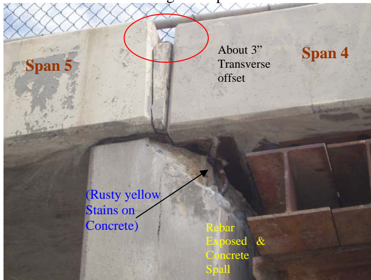
Figure 6 Concrete spalls and stains at the northwest corner of Pier 5 (note stains).
