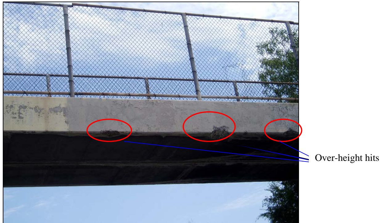
Figure 4 Damage to superstructure from over-height hits in Span 4
