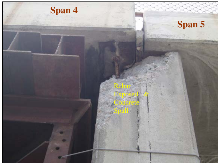
Figure 5 Concrete spalls at the southwest corner of Pier 5; note the evidence of corrosion on the dowel connecting the superstructure voided slab to the pier
