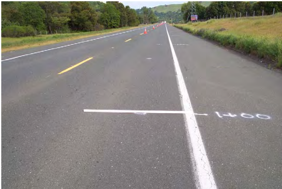
Pavement Condition within PES 5 (Rut Measurement with a 6-ft Straight Edge)
