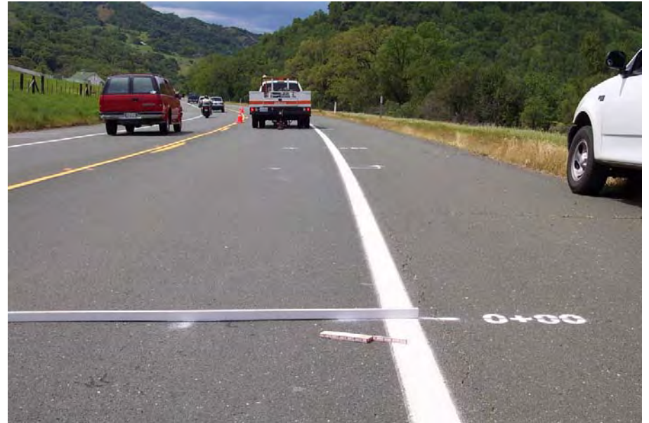
Pavement Condition within PES 3 (Rut Measurement with a 6-ft Straight Edge)
