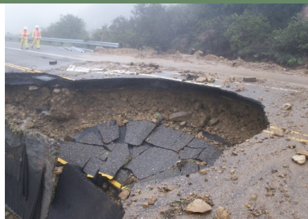
Landslide, Highway 154 in Santa Barbara County
