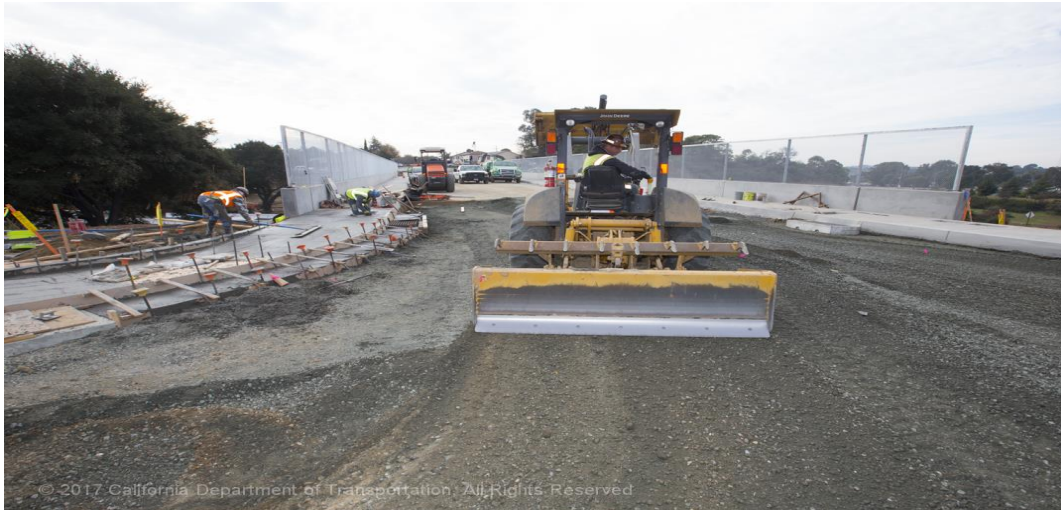
Grading of approaches to new bridge on Laurel Street. (Caltrans Photography, December 20, 2017)
