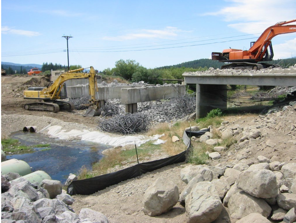
Figure 7-1. Clear Water Diversion Through Culverts with Bridge Removal on Gravel Pad, Sulpher Creek
