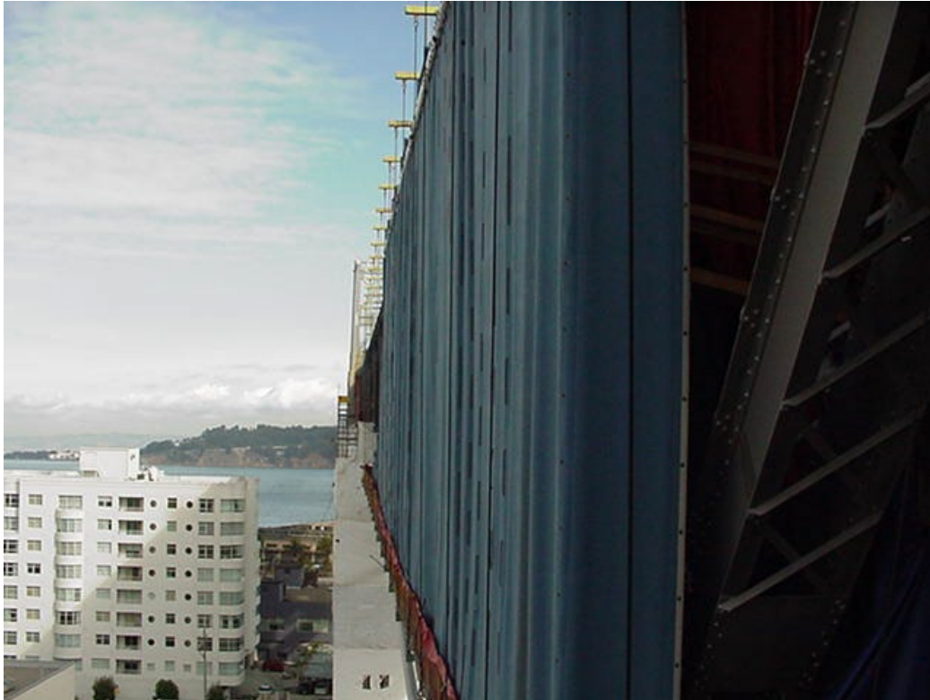
Figure 7-14. Sound Control Blanket on the Continuous Truss of Bay Bridge
