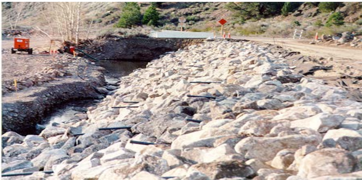
Figure C5-4: Half-ton RSP with Weep Pipe, District 10, East Fork Carson River Courtesy, Jim Racin, ESC, Office of State Highway Drainage Design, 1-97.
