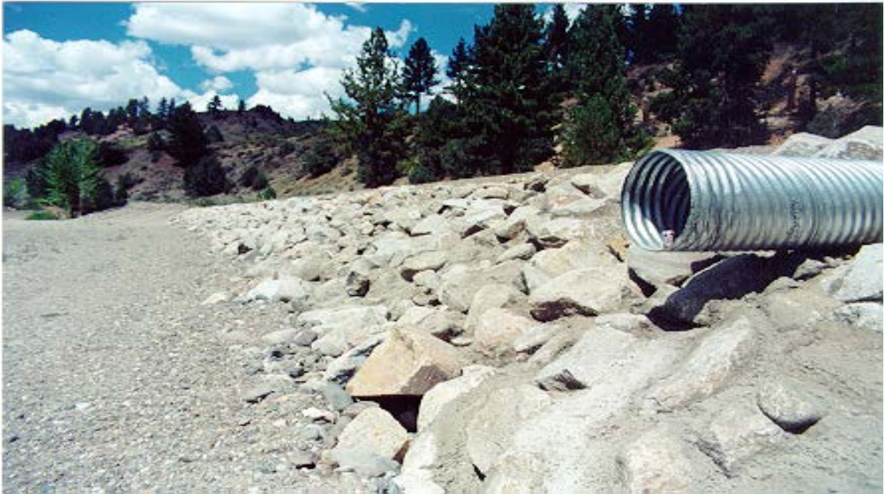
Figure C5-5: Grouted RSP, District 10, East Fork Carson River. Courtesy, Jim Racin, Office of State Highway Drainage Design, 1-97.
