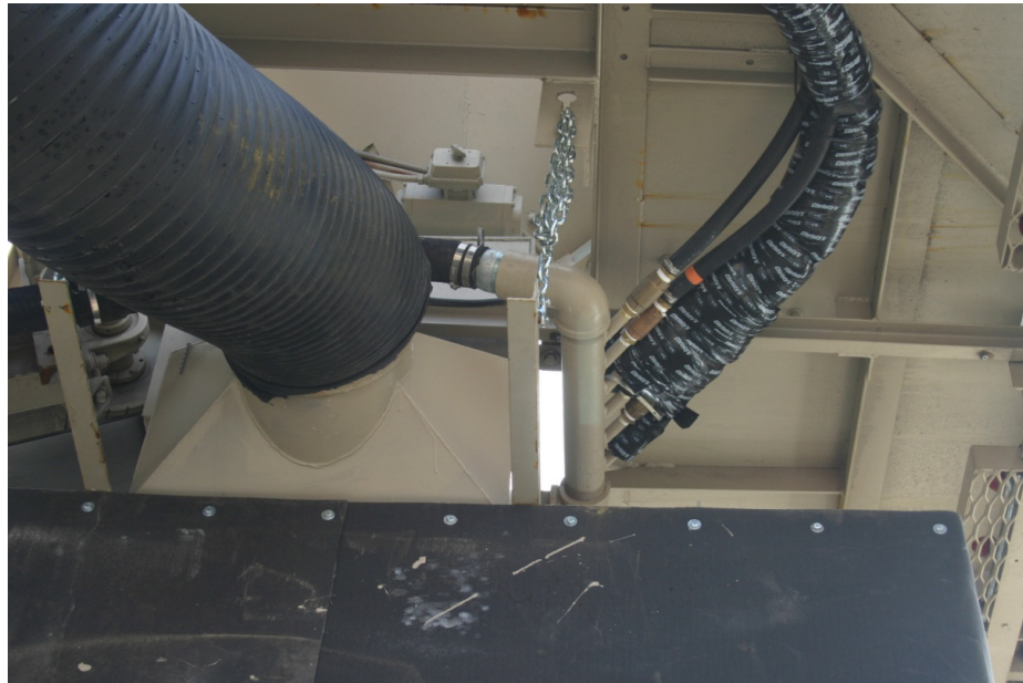
Figure 4-10. Manifold Where Liquid Admixture Enters the Stream of Batch Water.
