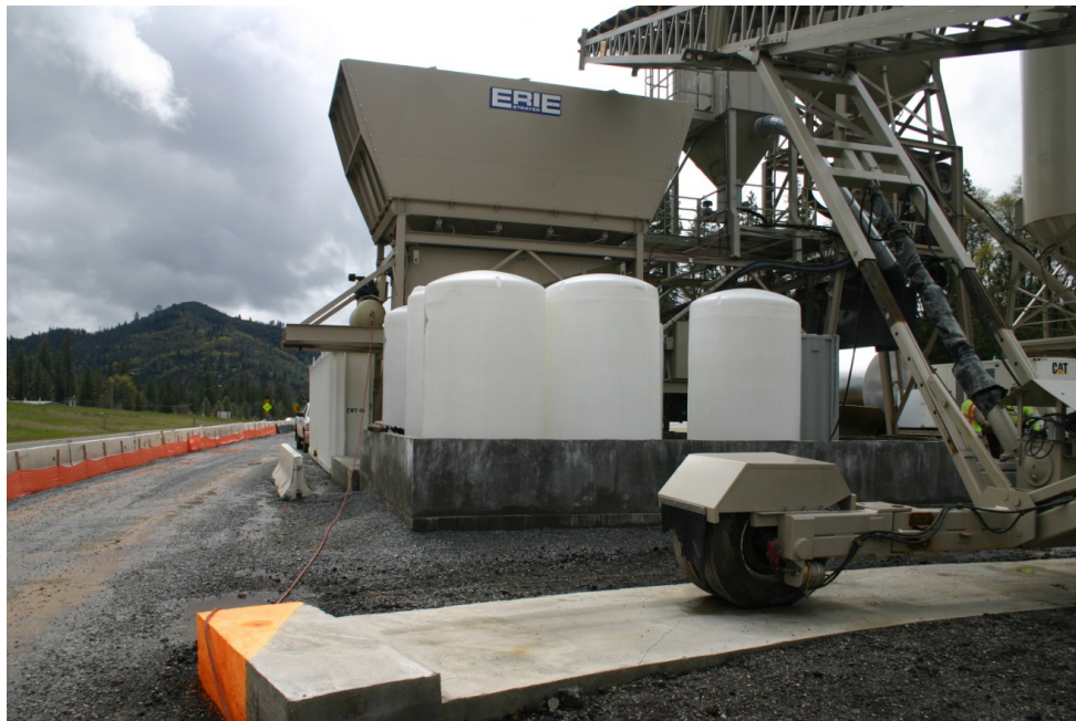
Figure 4-9. Liquid Admixture Storage Units.
