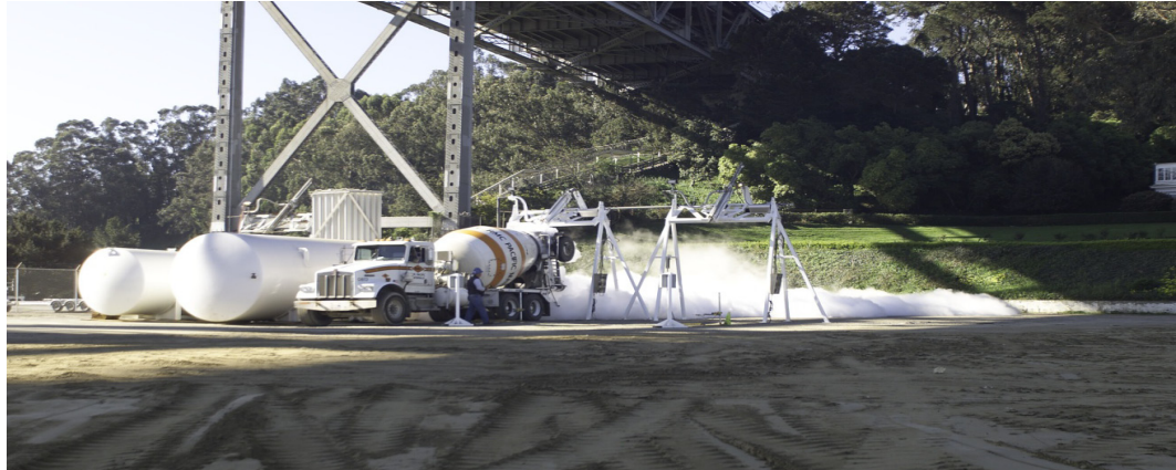
Figure 4-12. Liquid Nitrogen Being Injected Into a Transit Truck to Cool the Concrete.
