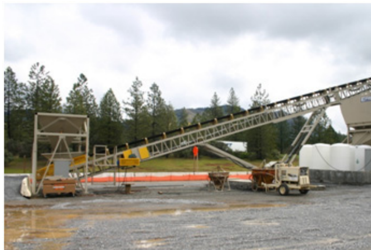
Figure 4-6. Weigh Hopper Under Aggregate Bins.
