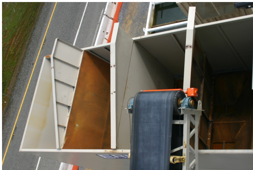
Figure 4-3b. Aggregate Storage Bins.
