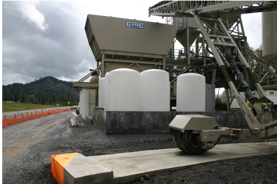
Figure 4-3a. Aggregate Storage Bins.
