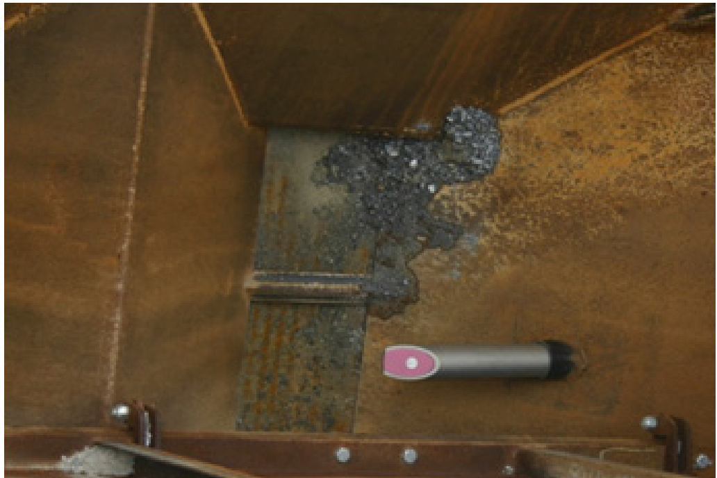
Figure 4-8. Moisture Meter at the Bottom of a Fine Aggregate Bin.
