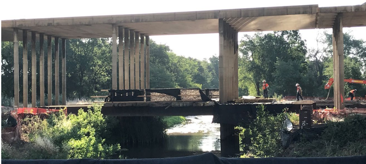
Figure 5-7. Trestle Type Protective Cover Over Waterway, Simerly Slough
