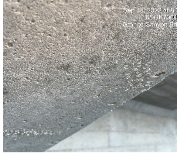
Figure 4. Silane Waterproofing Tested 7 Days After Application Depicts Proper Water Beading on Treated Surface
