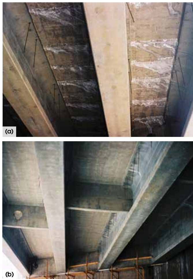
Fig. 6: Cast-in-place decks and spliced precast bulb-T girders on I-80 near Truckee, CA: (a) deck constructed without SRA; and (b) deck constructed with SRA (photos courtesy of Ric Maggenti)
