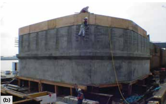
Fig. 7: Concrete footing jacket on the skyway portion of the new span for the SFOBB: (a) stay-in-place steel forms with headed studs; and (b) finished jacket, exhibiting no visible cracks (photos courtesy of Bill Lee and Ric Maggenti)
