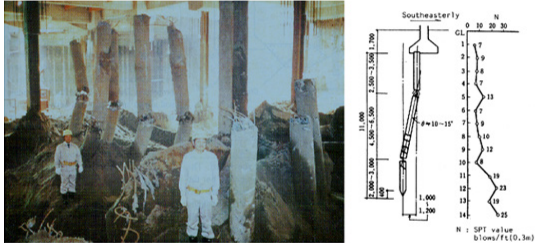
Figure 7 The NHK Building on piles that formed two pins during the 1964 Niigata EQ
